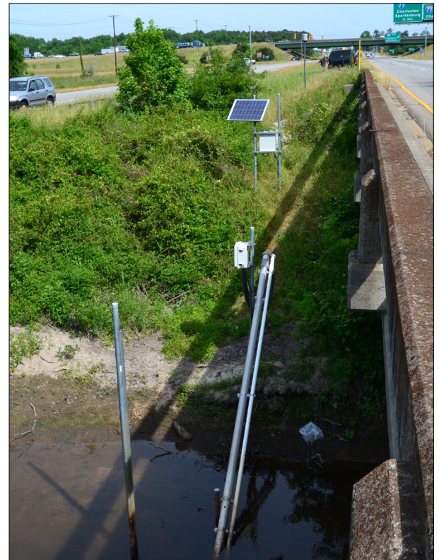
The GIL-C Monitoring Station
