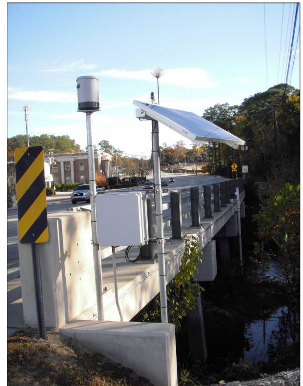
The GIL-A Monitoring Station
